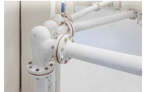
The Upper Occoquan Water Reclamation plant has gone 16 years without an elbow failure after installing short radius Smart Elbow® deflection elbows.
